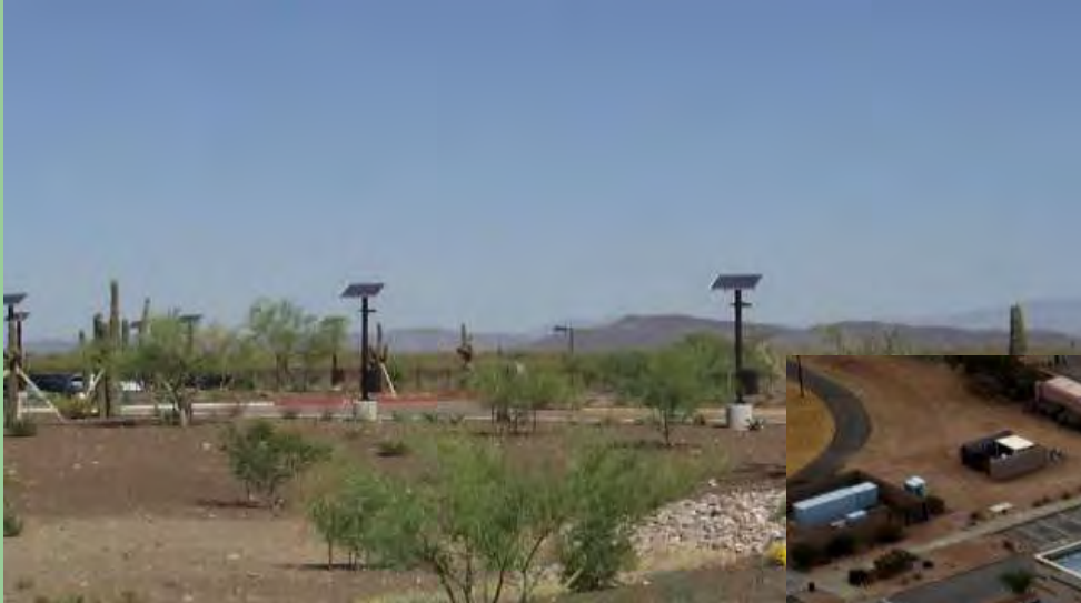
Parking lot lighting
