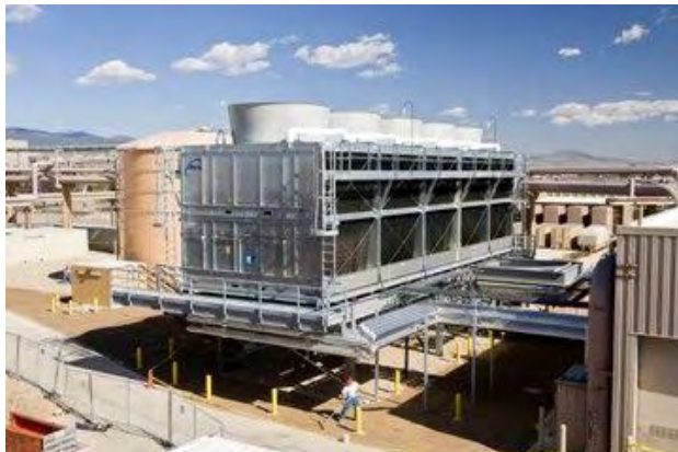
Cooling towers. Photo: IBM
