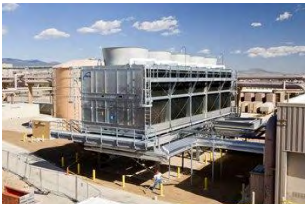
Cooling towers. Photo: IBM
